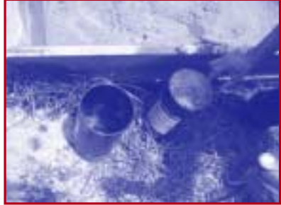
Poor quality concrete in Boaco
